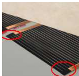
Insulate the copper lanes with duct tape or pvc tape
